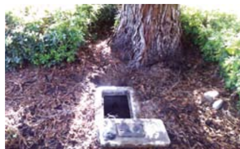
This tree was planted too close to the service box. As the tree matured, its roots damaged the service box, causing a leak.
